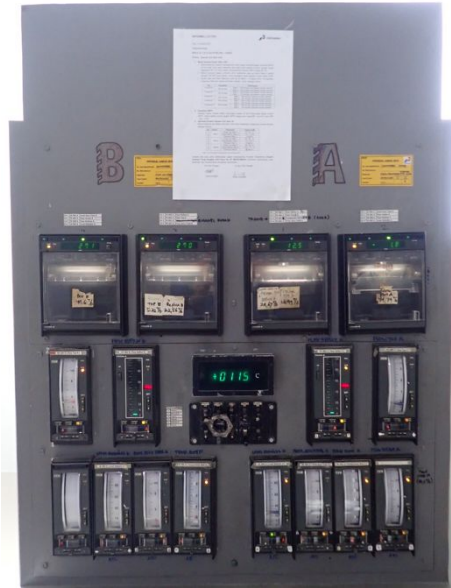
Discrete (single loop) controllers
