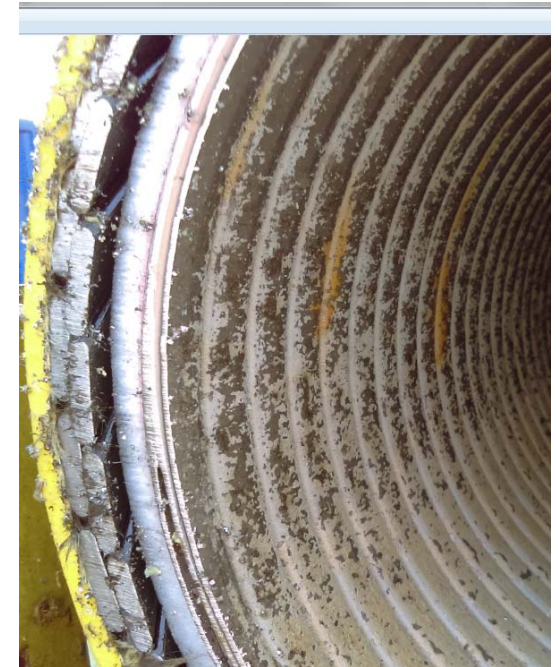
Water Injection riser with NORM's scale
