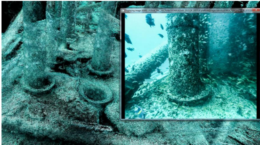
Conductor lack of Centralization
